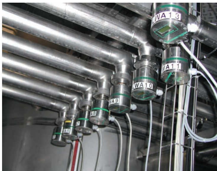
ILM-2 devices in a CIP-cleaning-circuit for phase separation of lye - acid - water.
